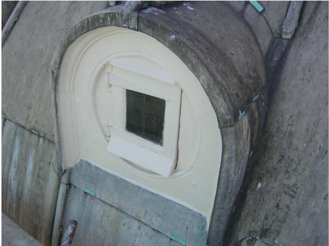
Repaired and redecorated timber casement window within main cupola roof. One of eight similar dormer windows.
