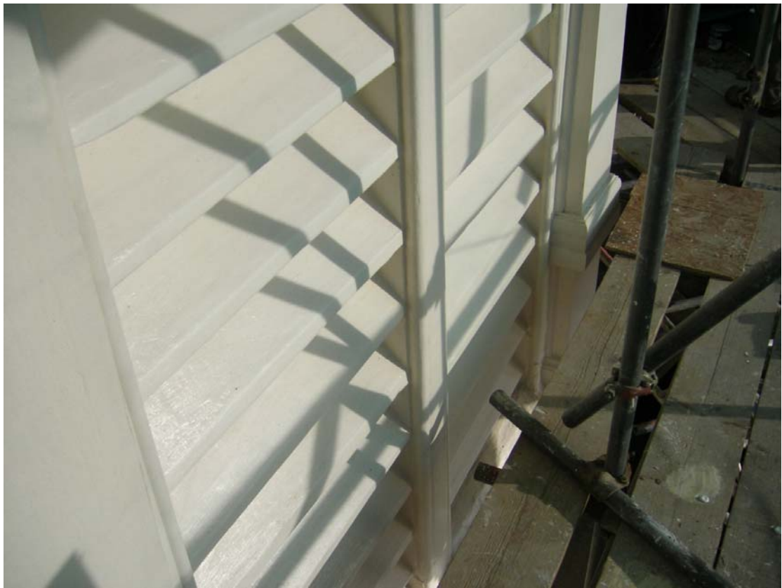
Louvres to the Belfry. Some of the louvres were decayed and have been replaced with new.
